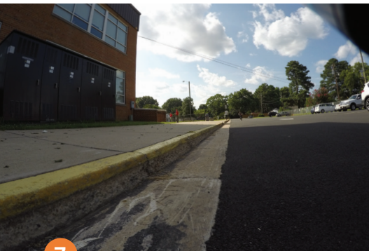
7 After paving, the curb and gutter section is functioning once again. Yellow paint on curb shows how high the pavement used to be.
