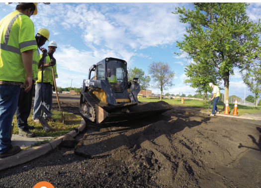
2 Gutters were filled with multiple layers of asphalt that had to be carefully removed to re-establish a functioning curb.
