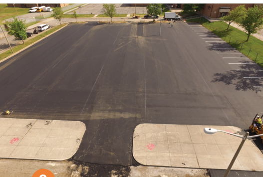
8 After the new FDR base is overlaid with a single lift of asphalt, the parking area is ready for stripping and immediate use.
