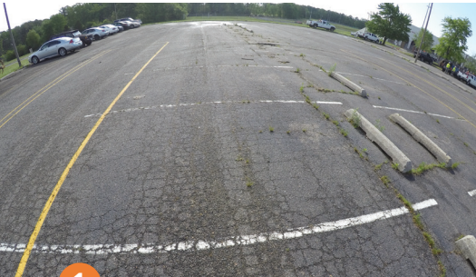
1 Despite multiple overlays, the deteriorated parking lots were needing more than a mill-and-fill approach.
