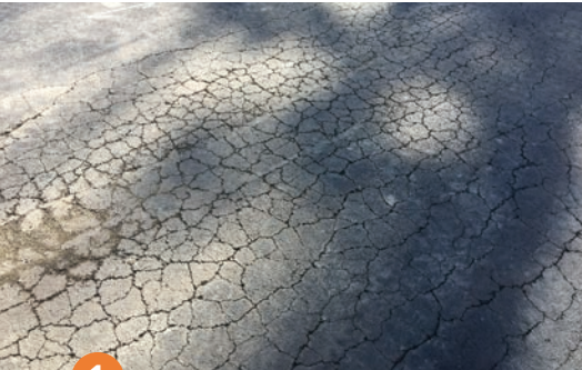
1 Prior to reclamation, the Westin's parking lot was riddled with alligator cracking, indicating an inadequate pavement structure
