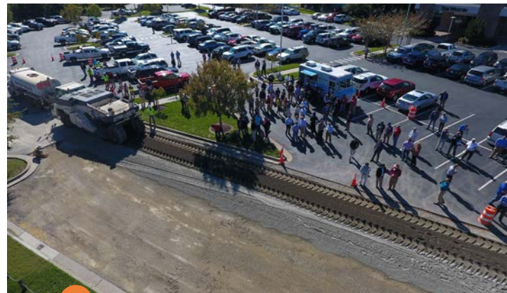
7 During the second pass, water was added through the head of the machine
