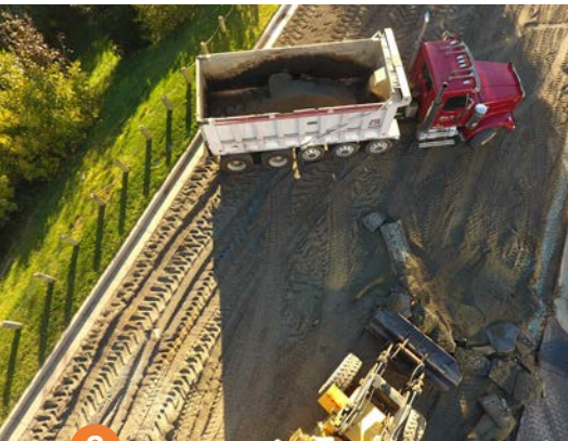
2 Removal of excess material after initial pulverization to allow 2.5 inch overlay to match existing curb line
